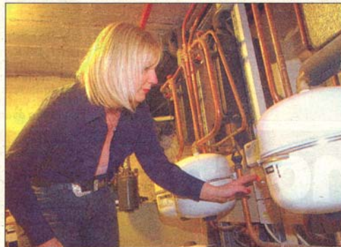
ECO-FRIENDLY HOTEL: Claire Smith switches on the new solar energy boiler at the Number One hotel
